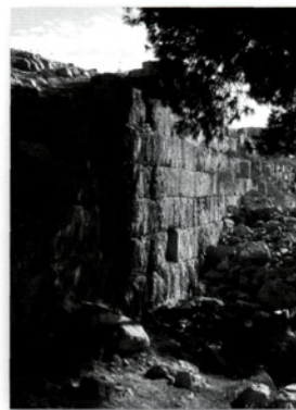
The fortifications on Jabal al-Qal'a, overlooking Amman, have been damaged by earthquakes and repaired several times. The relatively weak fortifications here, on the west side of the site, have buttresses or rudimentary towers that protrude only a short distance from the main wall. (Author's photograph)
